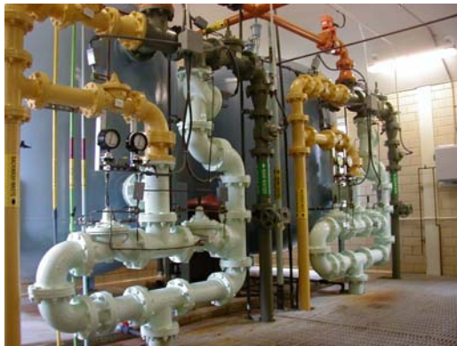
Brunswick & Topsham Water Treatment Plant
