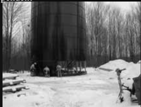
South Rome, New York Tank Size - 25 dia. x 120 high Tank Capacity - 450,000 Gallons Constructed - January 2004
